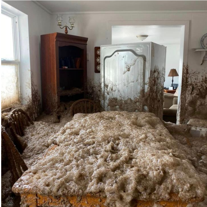
In Port-aux-Basques, N.L., New Glasgow, N.S., and Neils Harbour, N.S., Hurricane Fiona left its mark on Atlantic Canadians' homes last September. It is estimated
