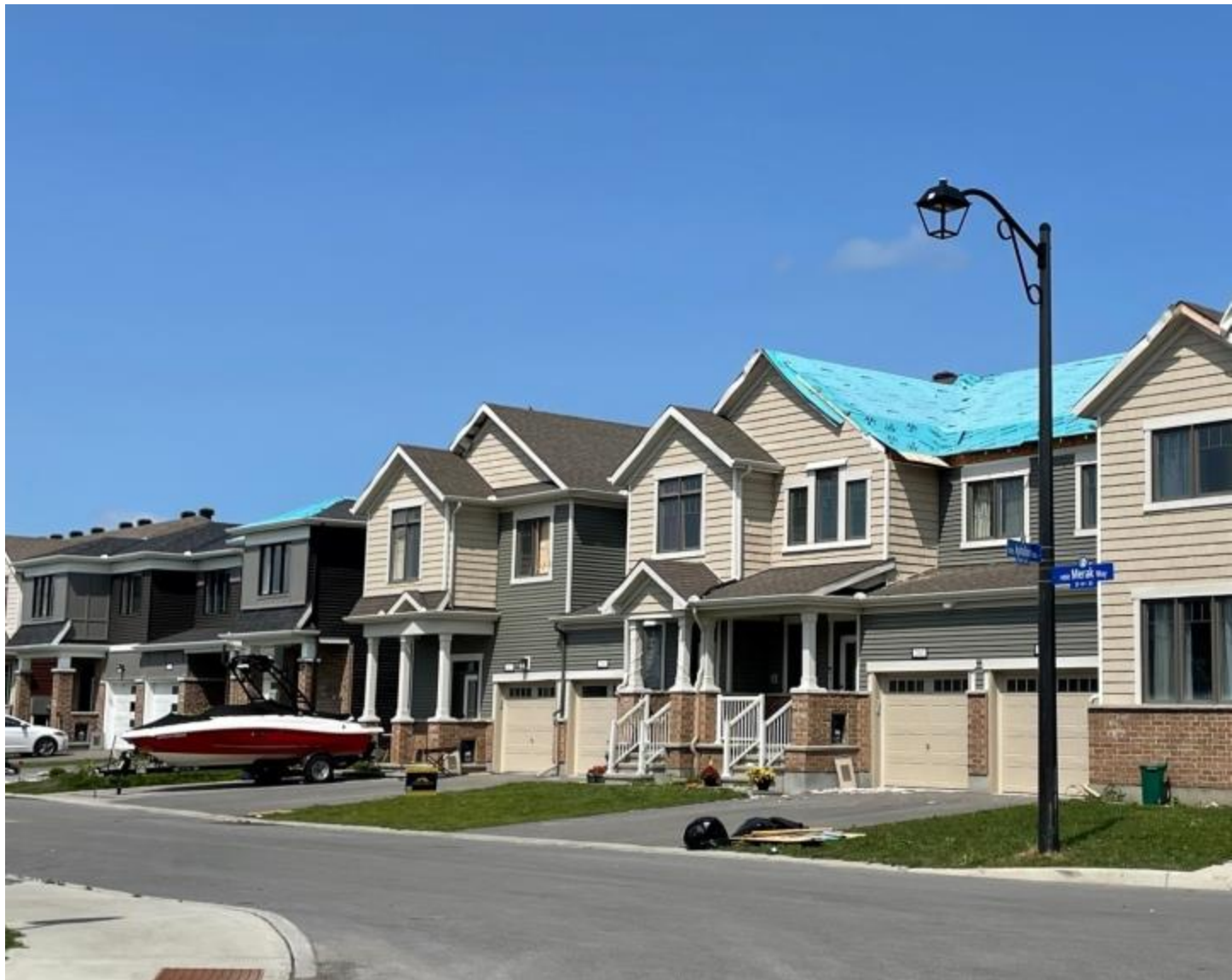
A tarp covers a damaged roof on Metal Way in Barrhaven, one day after a tornado ripped through the area. (Peter Szperling/CTV News Ottawa)
