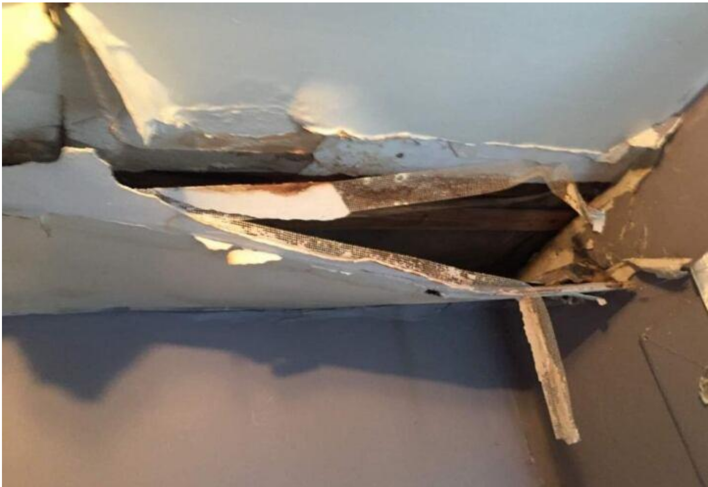
The roof above one of the rooms in Prosper's home caused the ceiling to collapse and water to penetrate the walls. (Submitted by Melissa Prosper)
