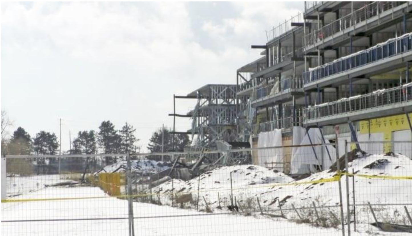
Upper Vista Welland partially collapsed again on Sunday, after previously partially collapsing on Feb. 18. (Joseph Burd/CBC)
