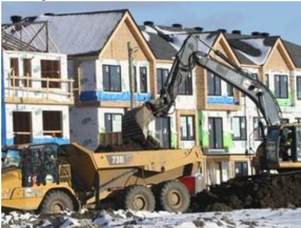
A construction crew works on new houses in Barrhaven. PHOTO BY TONY CALDWELL /Postmedia
