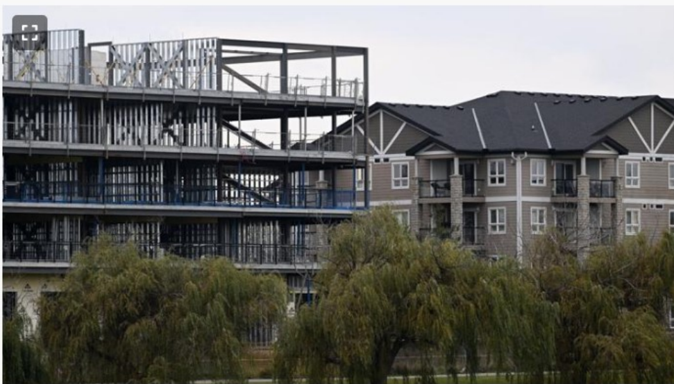
Work on the fifth floor of Evertrust Developments' Upper Vista Welland project is underway. Also seen is Seaway Pointe condominiums next door.
